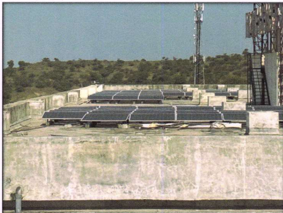
Photograph of Solar PV Plant:
