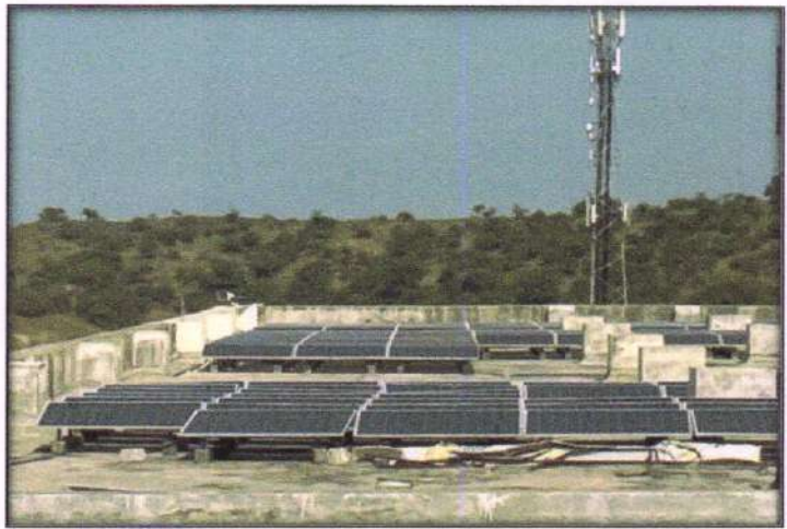
Photograph of Solar PV Plant:
