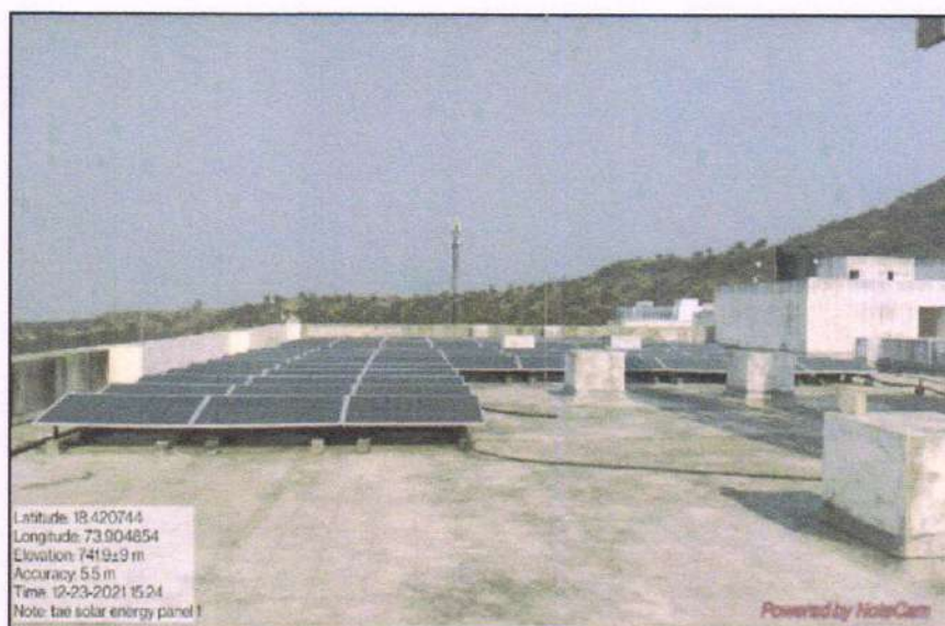
Photograph of Roof Top Solar PV Plant:
